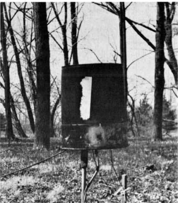
The complete tuning unit is installed inside of the paint pail. A tight fit prevented damage during a recent flood. The 160-meter radials are secured to the vertical support pipe by a hose clamp.
